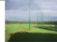
7 Metre High Golf Net Fencing Applied as per planning drawing reference: 570 - 004K - Proposed Boundary Treatment Plan
